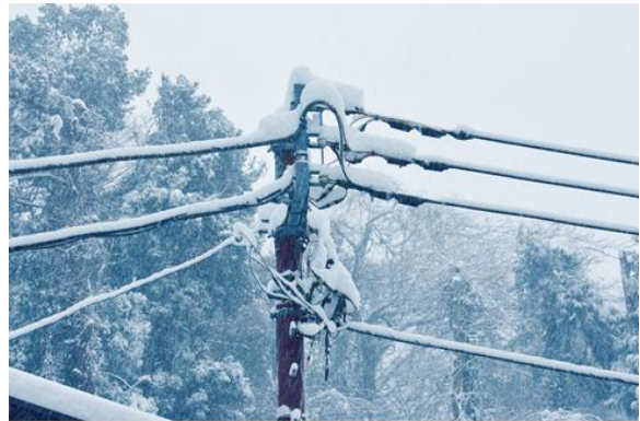
Mitigating ice accumulation on power transmission lines will help prevent outages
